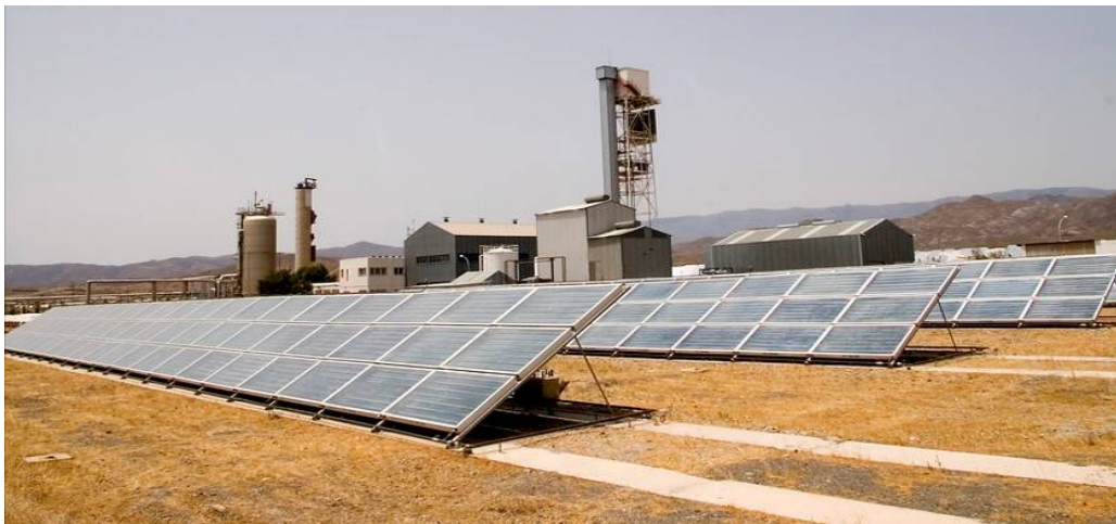
AQUASOL solar distillation plant at PSA
