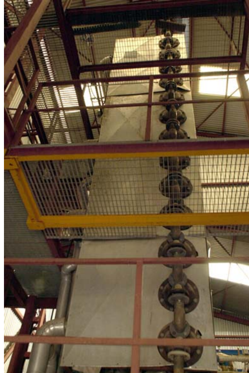
AQUASOL solar multi-effect distillation plant at PSA
